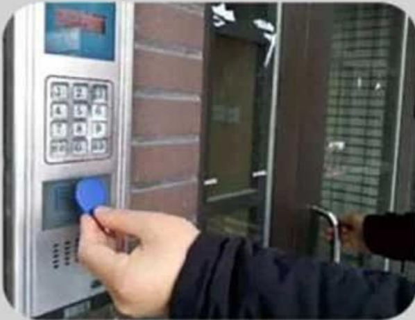
Door Access Control
