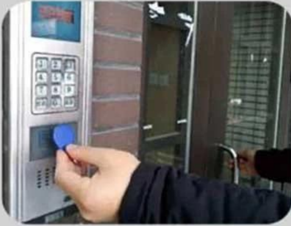
Door Access Control
