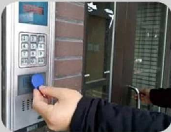
Door Access Control
