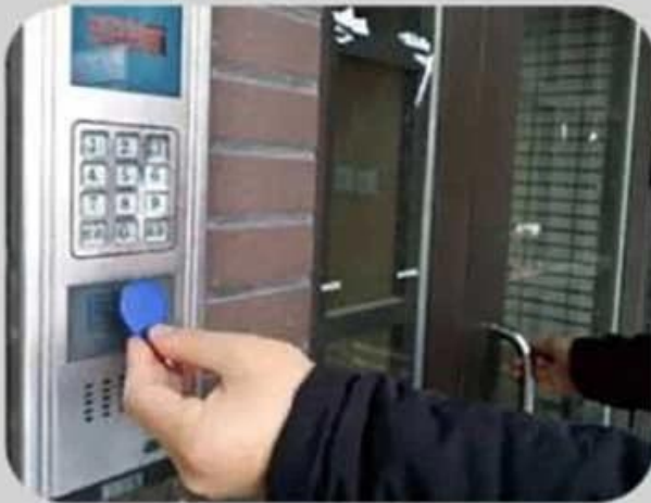
Door Access Control
