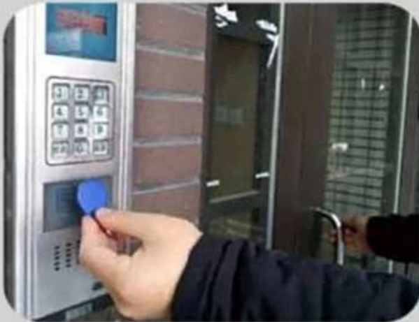
Door Access Control
