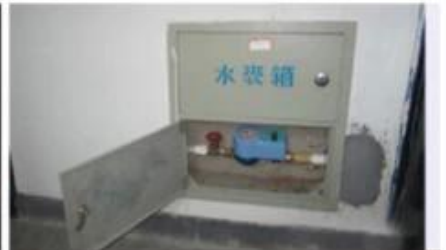
WATER METER BOX
