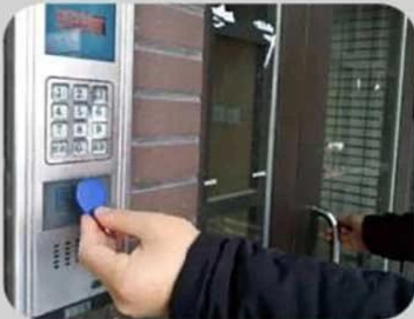
Door Access Control
