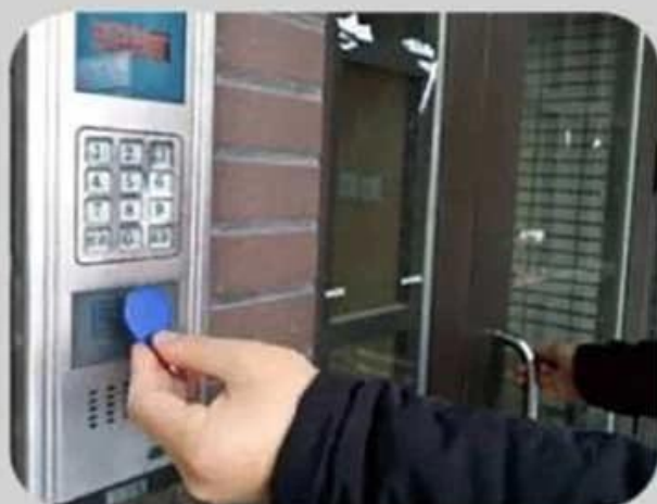
Door Access Control
