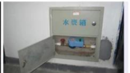
WATER METER BOX
