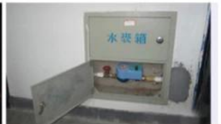
WATER METER BOX
