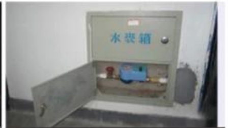
WATER METER BOX
